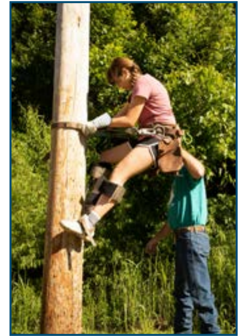
After watching G.R. Kirkpatrick (Cimarron Electric Co-op) demonstrate the safe way to climb poles, Baylee Oister takes her turn at climbing.
